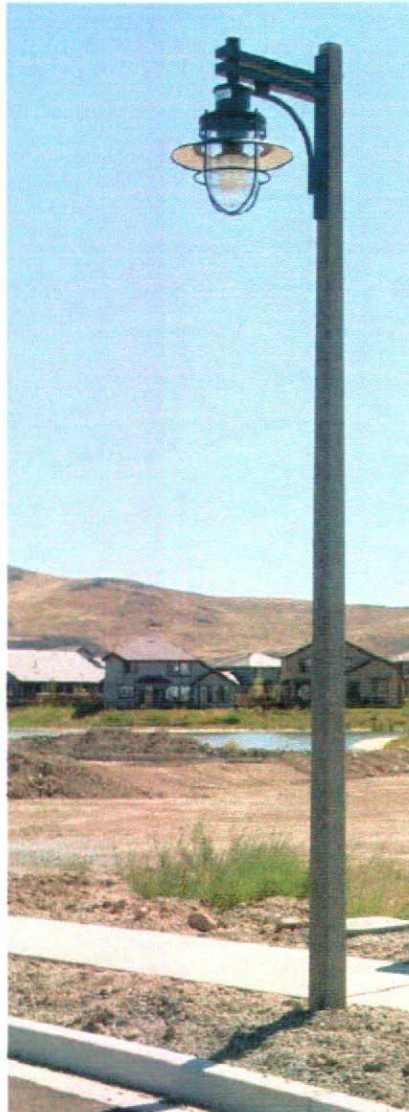
Figure 2-56 Disc Drive and Galleria Parkway Street Lighting
